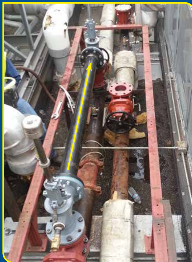
DUAL 6" x 4" LINE STOPS W/ 4" BYPASS PIPING OFF LINE STOP HOUSING
