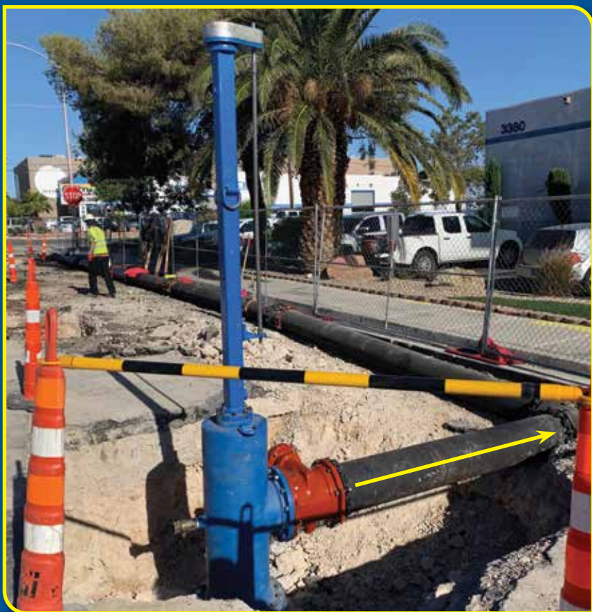
DUAL 24" x 16" LINE STOPS W/ 12" BYPASS PIPING OFF LINE STOP HOUSING
